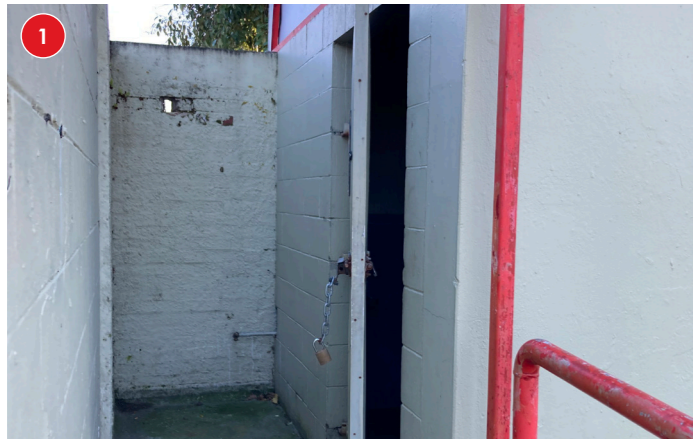
Existing public toilets in poor condition with entrapment risks.
